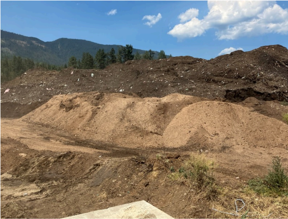
Photo 3. Compostable and recyclable materials, that have gone through Schedule 2 and 3 of OMRR, storage area.
