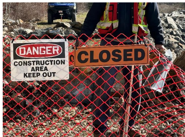
All access is closed with fences and signs.
