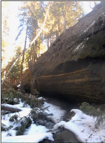
Photo 2: Erosion below 2809 Caen Road (looking downstream).
