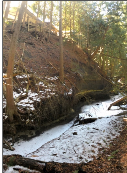
Photo 5: Looking across at erosion below property No. 2827 from bench across.
