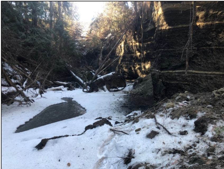
Photo 1: Looking upstream at culvert outlet and erosion.
