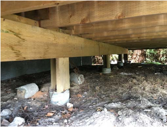
1-2x10 Post supporting ledger board & 2x10 joists, fastened to 4x4 post on 8" conc. columns
