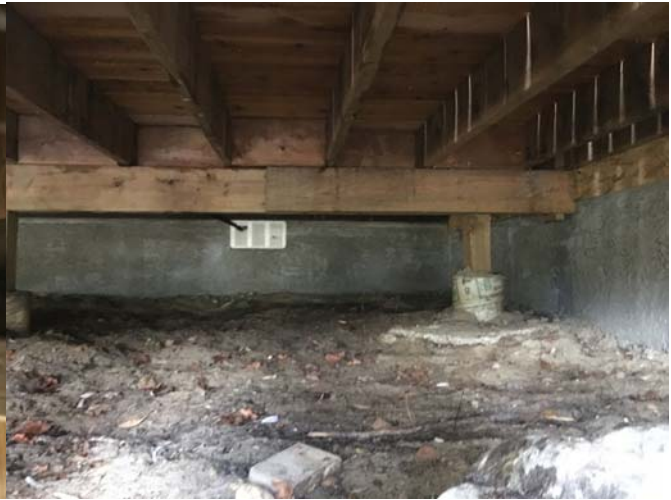
2 ply – 2 x 8 Beams supporting 2x 8 Joists with Scabbed on 2 x 8 to create a ledger board
