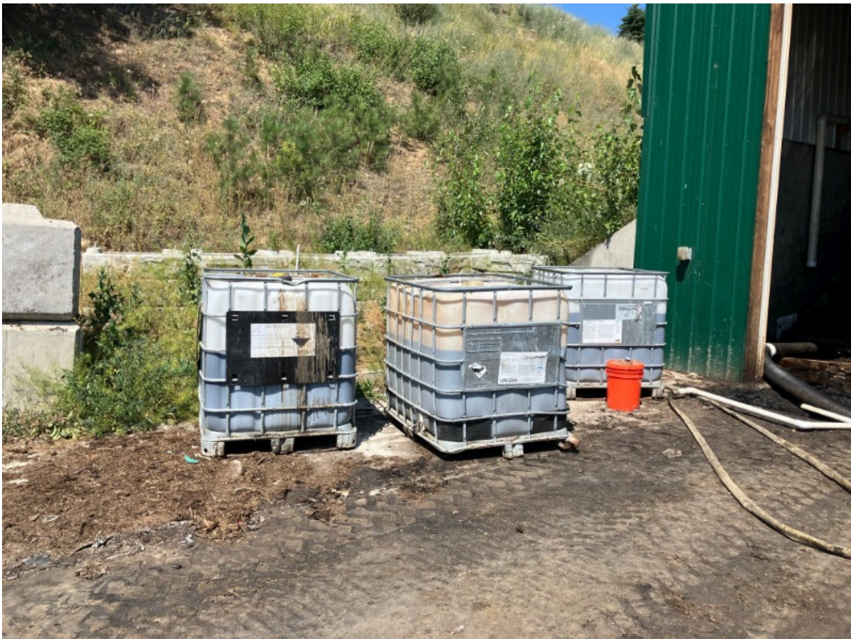
Photo 4. 4500L leachate collection system Facility recycles the leachate back into the composting process.
