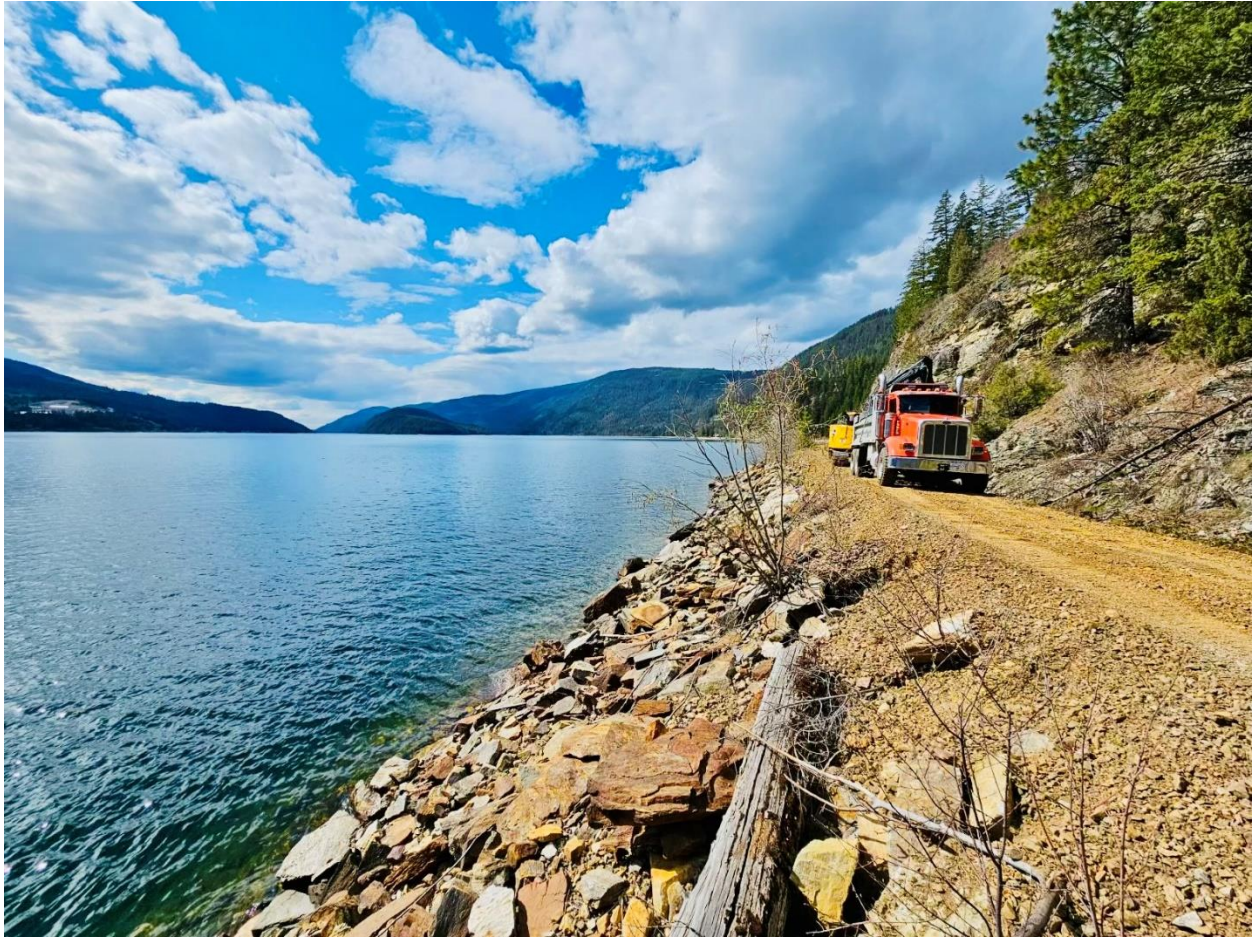
Splatsin team prepare rail bed ready to receive aggregate at north end of Mara Lake (Km 1.5-4.5)
