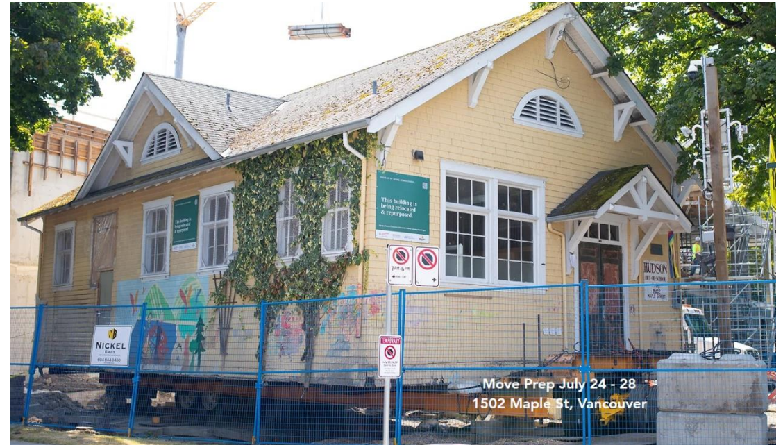
Relocation of Little Yellow School House, Squamish Nation Repurpose Project, From: renewaldevelopment.ca
