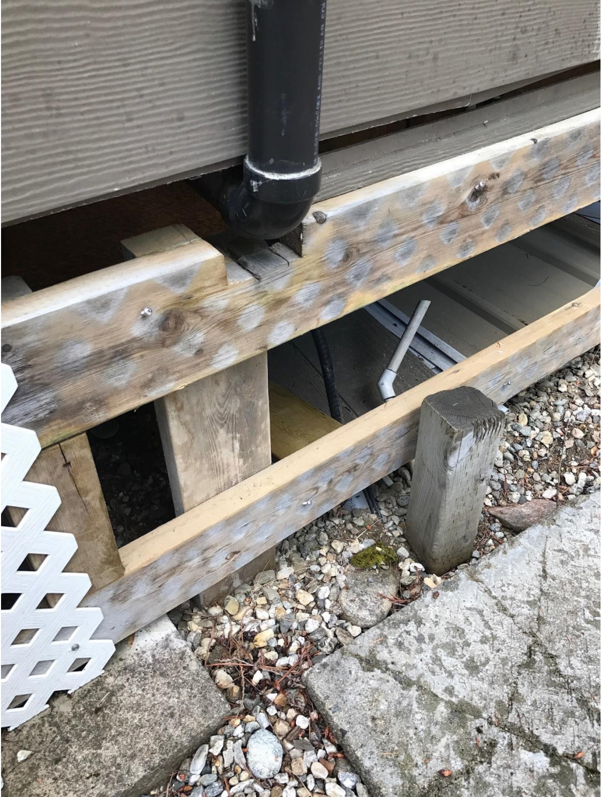
View showing water line connected to the bunkhouse severed
